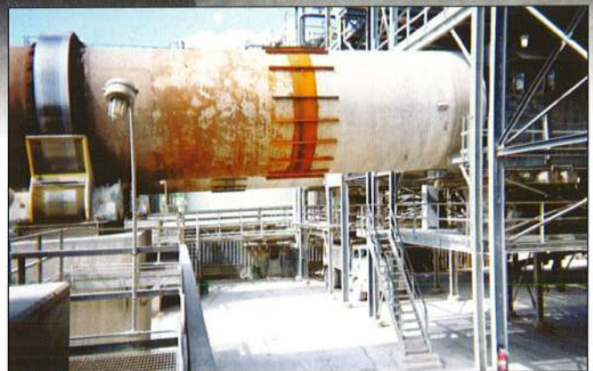
Figure 1. Reinforced shell: this practice should be avoided.
