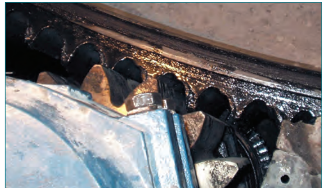
Figure 9. Very severe gear profile wear meshing with newer pinion. This gear should be replaced as soon as possible.
