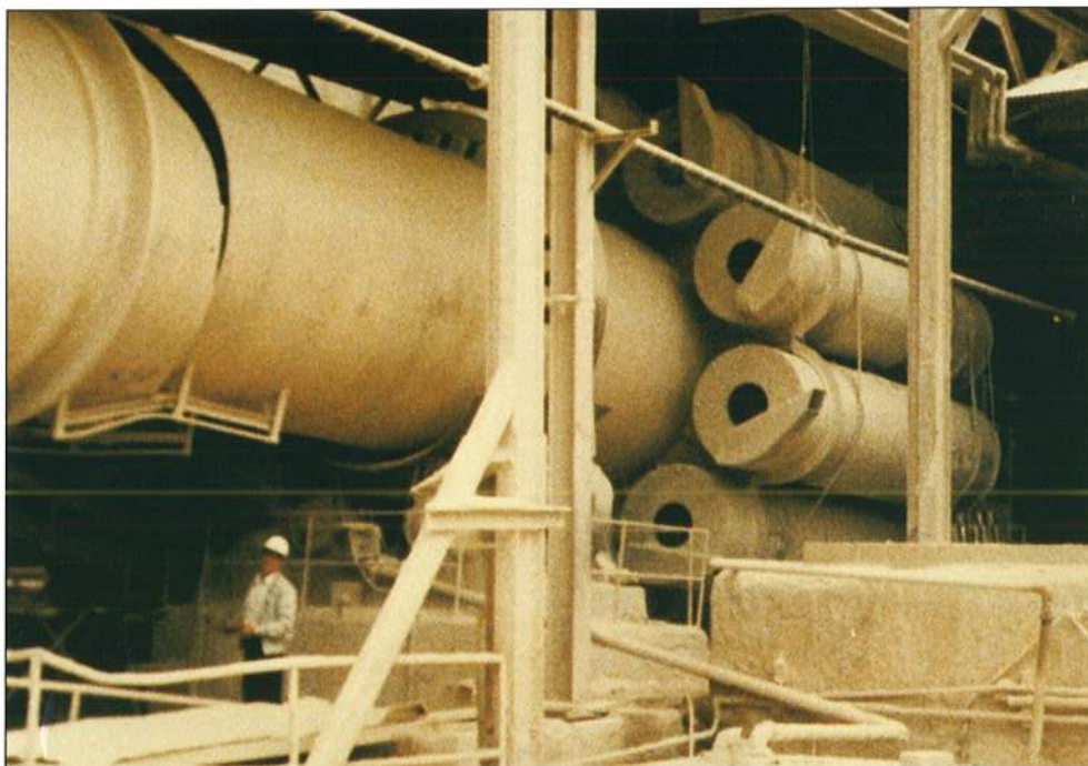
Figure 1. Catastrophic kiln failure.
